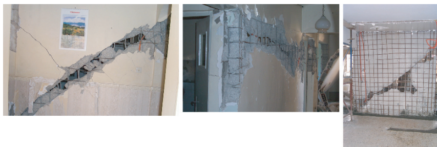
Fig. 3.4.3 Details of the structure. Crack on the longitudinal shear-wall at first floor (left), horizontal crack on the longitudinal shear-wall at first floor (center) and steel reinforcement of longitudinal shear-wall jacket (right)
